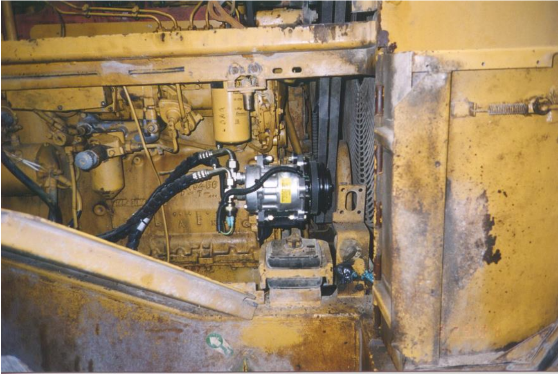
Compressor and mount in place.
